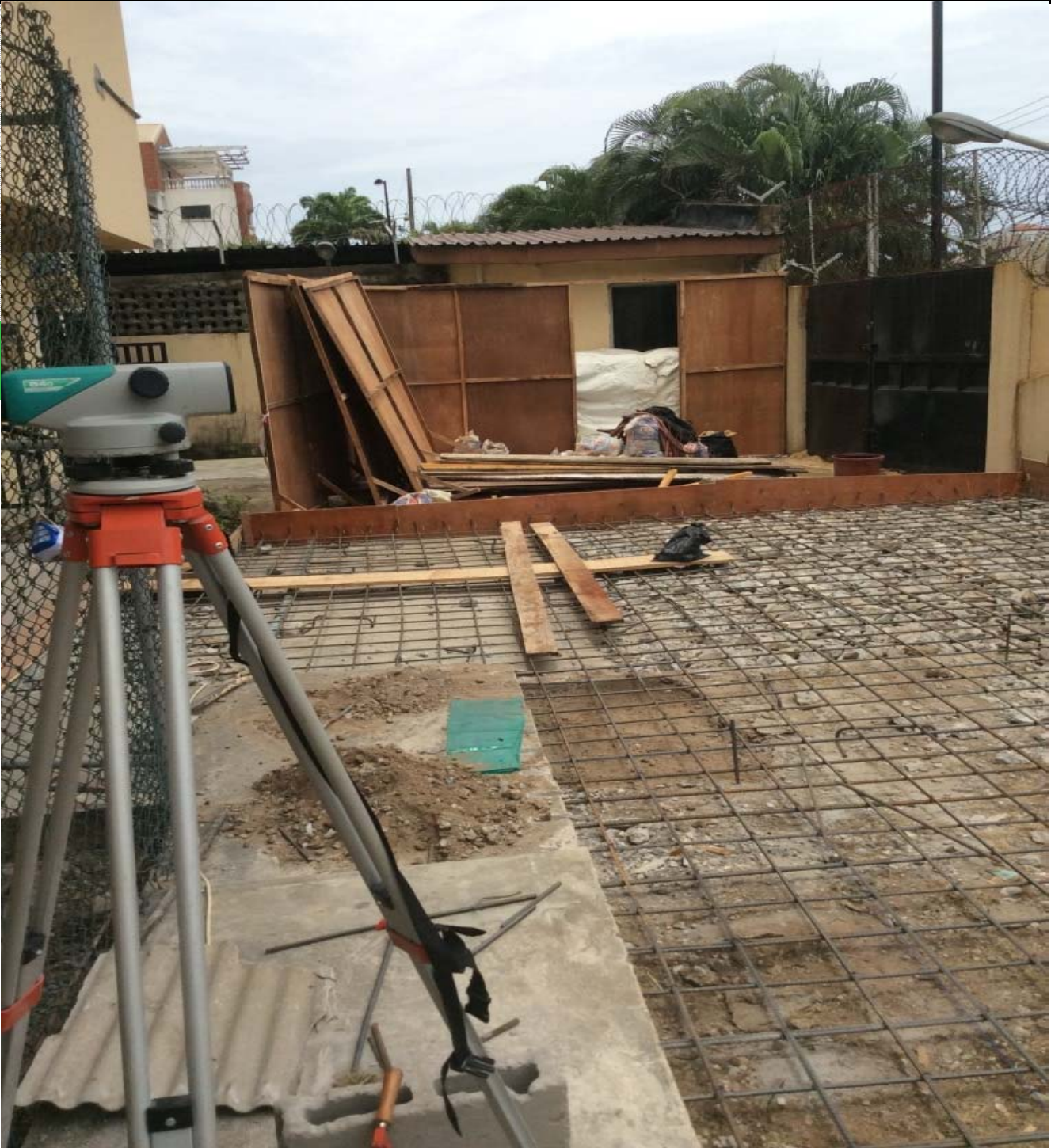
Construction of a Concrete Floor to Support an onsite Fabrication of Sound and Waterproof Portacabins - Association Francaise de Nigeria (French School), V/I, Lagos
